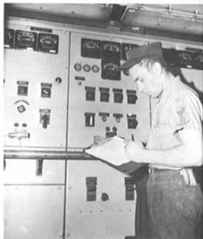
EN3 Bray takes hourly readings on ship's service generator board.
